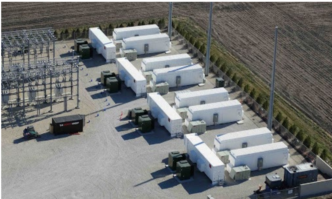
FIGURE 7-6 A STOCK IMAGE OF A SIMILAR DEVELOPMENT WITH AN ON-SITE SUBSTATION AND BESS.
