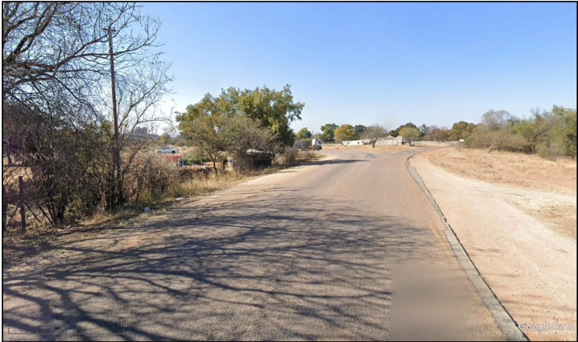
D114 approach to R565 lacks signage and is confusing giving the impression that one could possibly turn right.
