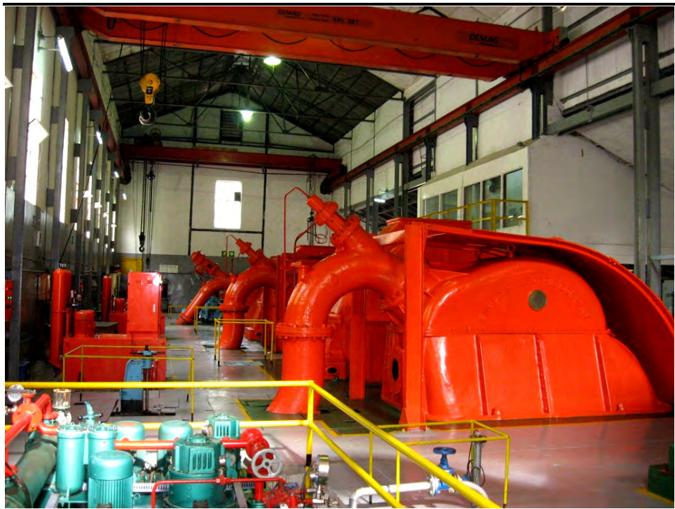
Figure 4.23 Existing Mulungushi Powerhouse: Internal View
